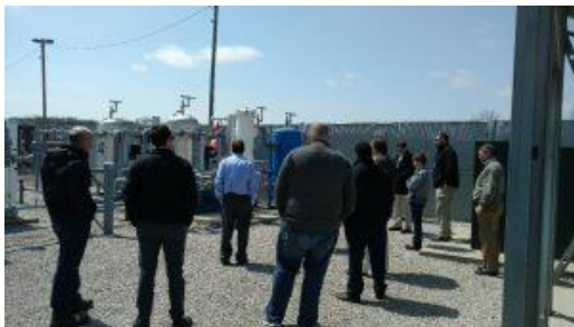
Here, the OMA's Sustainability Peer Network views the CNG compressor at SmithFoods Inc., Orrville.
