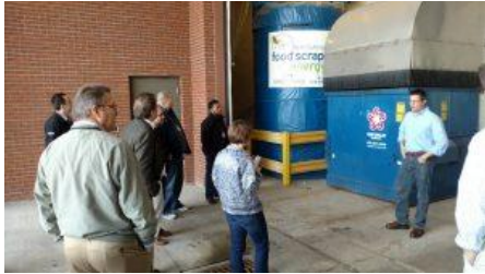
The OMA's Sustainability Peer Network tours The J.M. Smucker Company Grind2Energy installation.
